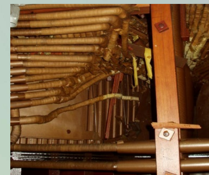
Displaced internal connections
