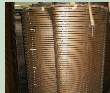
Damaged main winding
