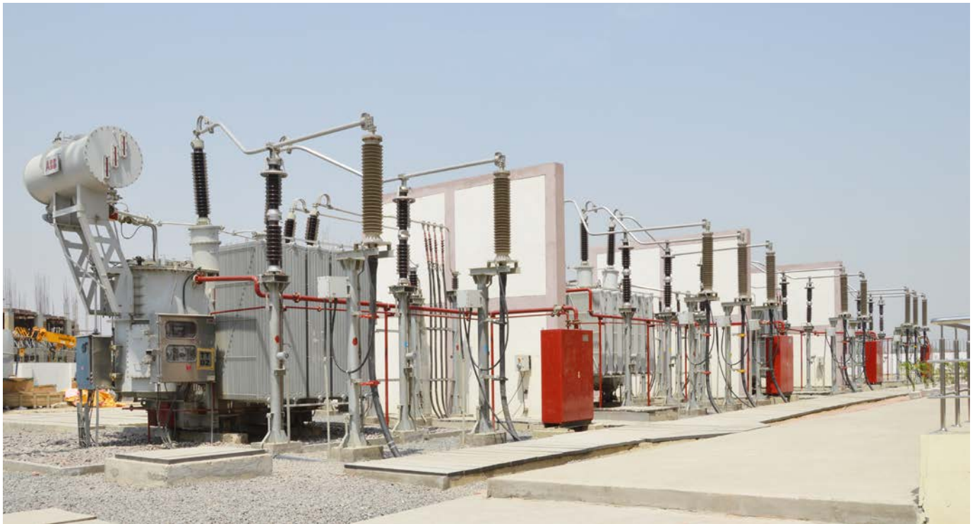
Figure 4. An array of four ABB trackside transformers installed by Indian Railways.
