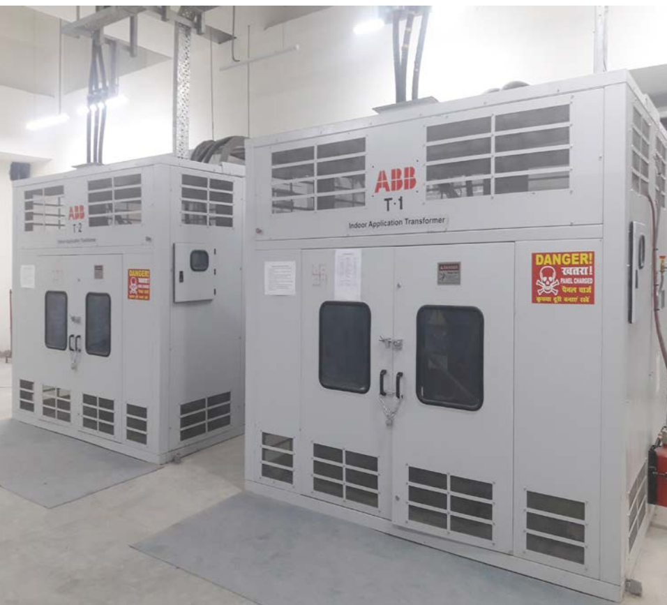
Figure 5. Dry-type transformers are ideal for underground or enclosed applications.
